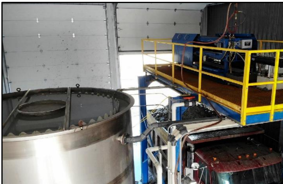
Stainless Steel Gravity Clarifier
